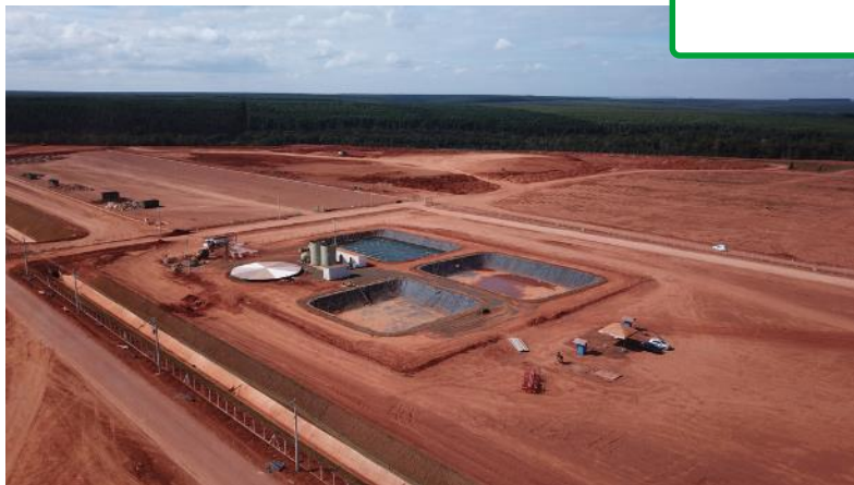
Temporary water and effluent treatment plant
